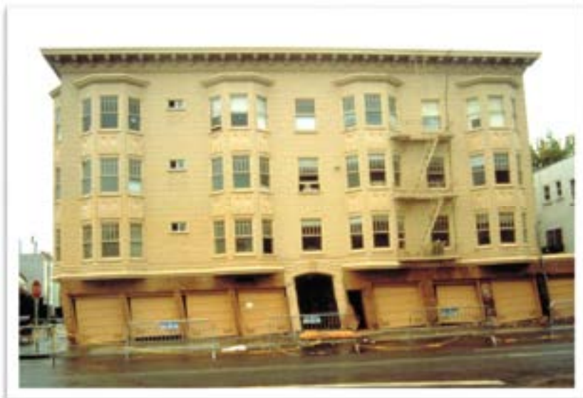
Fig.3.6. Clădire civilă cu nivel slab pentru garaje la parter, San Francisco, California, cutremurul Loma Prieta, 17 oct 1989, seism 6,9 Richter, National Information Service for Earthquake Engineering (NISEE), University of California, Berkeley
